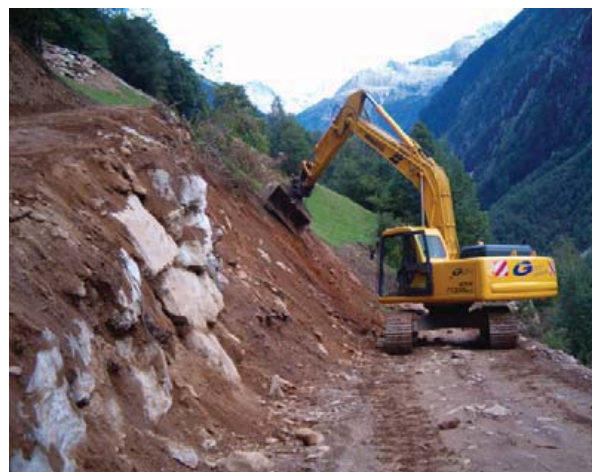
Fig. 7. Finisarea taluzelor cu excavatorul Performing the suitable angle of embankments with the excavator
